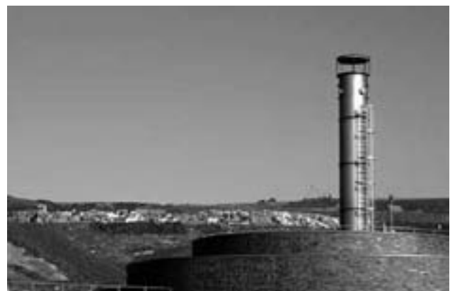
Fig. 4: Flare system at a landfill
